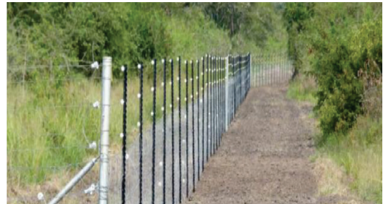
Plate 1. An electric fence limiting elephant crossing from PAs into villages (Credit: RDB, Rwanda)
